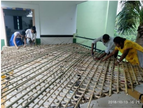
Progress in completion of Bamboo wall 1 under the mentoring of Ar. B.Amulya on 12-10-2018 @E210 - School of Architecture
