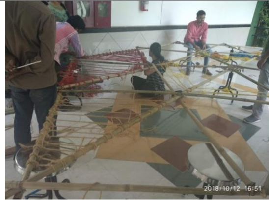
Frame work for roof done by students with the help of skills men and faculty on 12-10-2018 @E210 - School of Architecture
