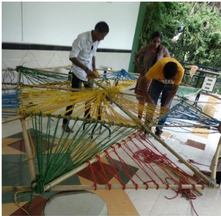
Students weaving the roof pattern with coconut foir on 13-10-2018 @E210 - School of Architecture
